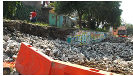
Figure 11. Slumped masonry retaining wall
