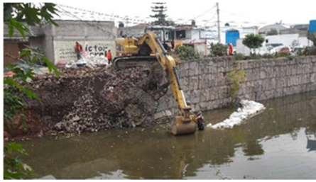
Figure 10. Slumped canal masonry side wall
