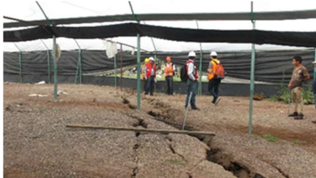
(a) Ground cracks inside a nursery
