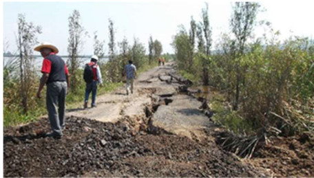
(a) Failed causeway segment
